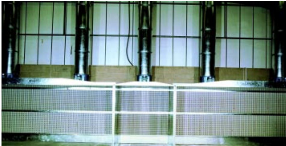
2 x 6.6 metre and 1 x 2.75 metre wide Sirocco spray booths
