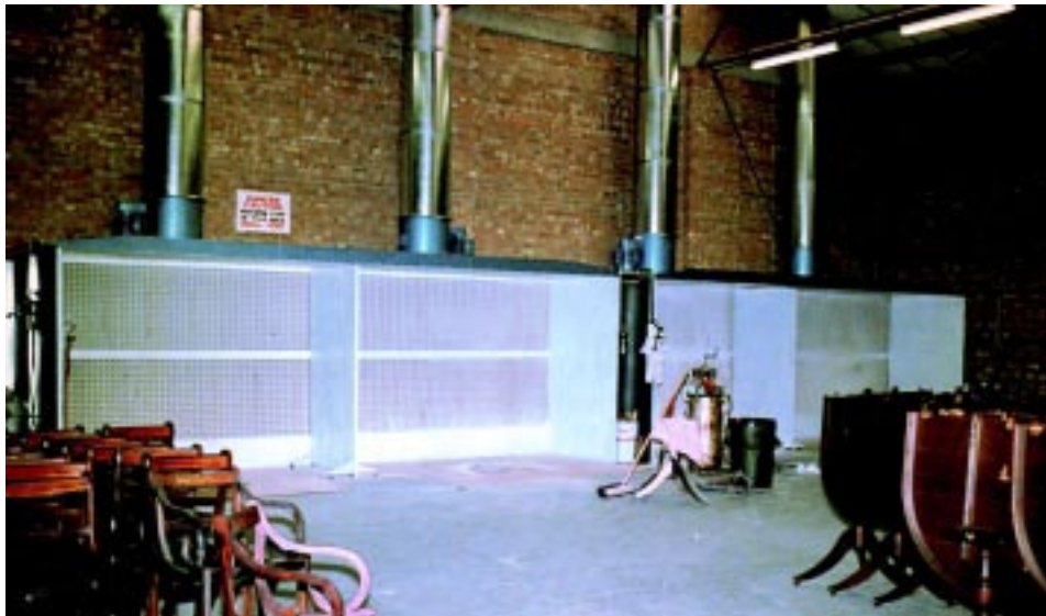
2 x 6.6 metre wide Sirocco spray booths
