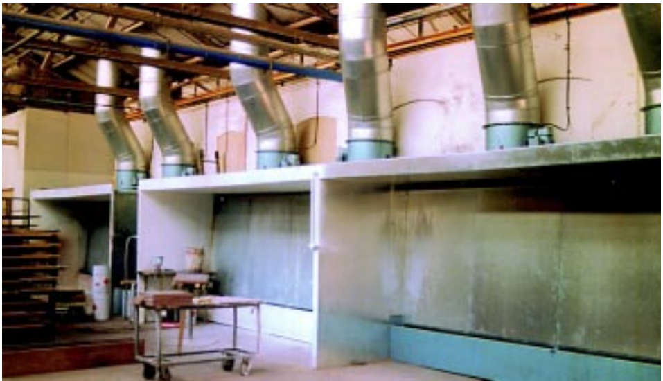
3 x 5.5 metre wide Cascade spray booths
