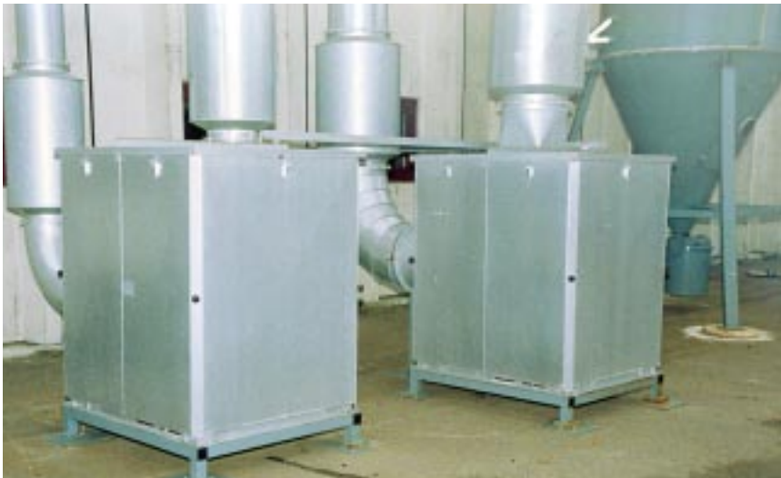
2 x 45 kW fans mounted within acoustic housings and incorporating duct silencers, used to extract metal grinding dust.
