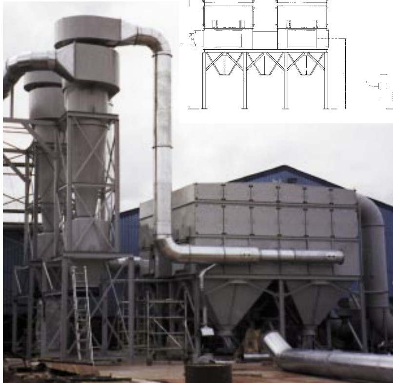
Valley Hopper – Large capacity filter units with Valley Hopper collection facility, mounted on supporting steelwork
