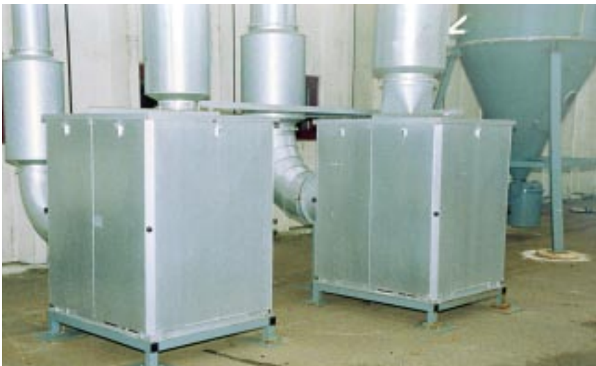
2 x 45 kW fans mounted within acoustic housings and incorporating duct silencers, used to extract metal grinding dust.
